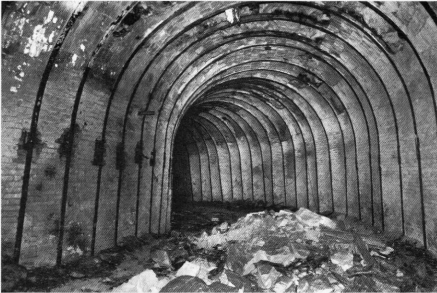
One of the main tunnels. Note the hooped construction and the arched railway lines used. Photo Tony Page
